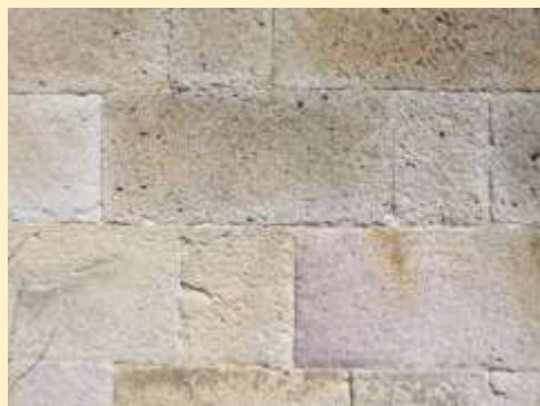
The warm hues of Pentewan Stone bring character and quality to even plain stonework.
