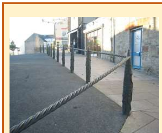
New ironwork and granite paving on Biddicks Court as part of street improvement scheme
