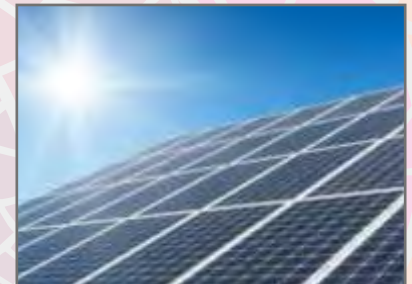
Solar Panels White River Place
